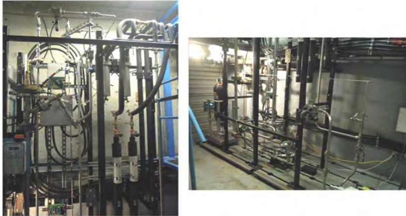
Figure 4-16: Upper and lower views of the heat transfer test facility with carbon dioxide flow
