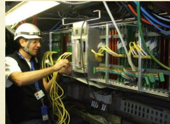
Installation DCal au CERN
